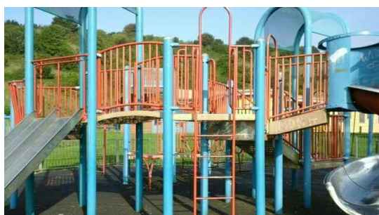
Image 3: Photograph of multiplay equipment at Whitehawk Senior, taken as part of the Annual Inspection
